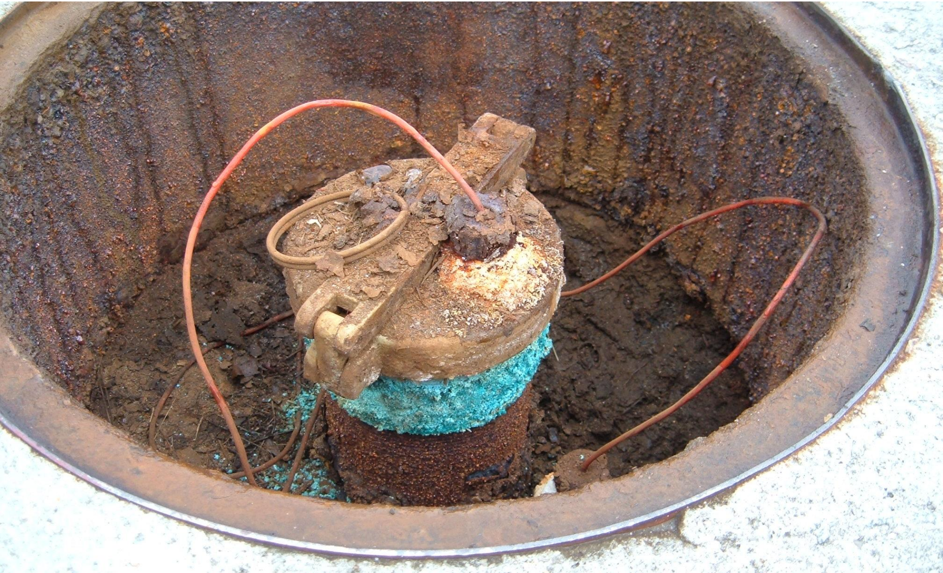
Evidence of vapor leaks
