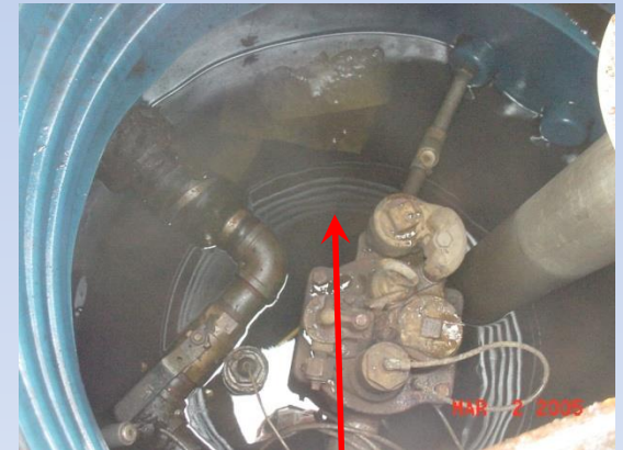
Gasoline in sump
