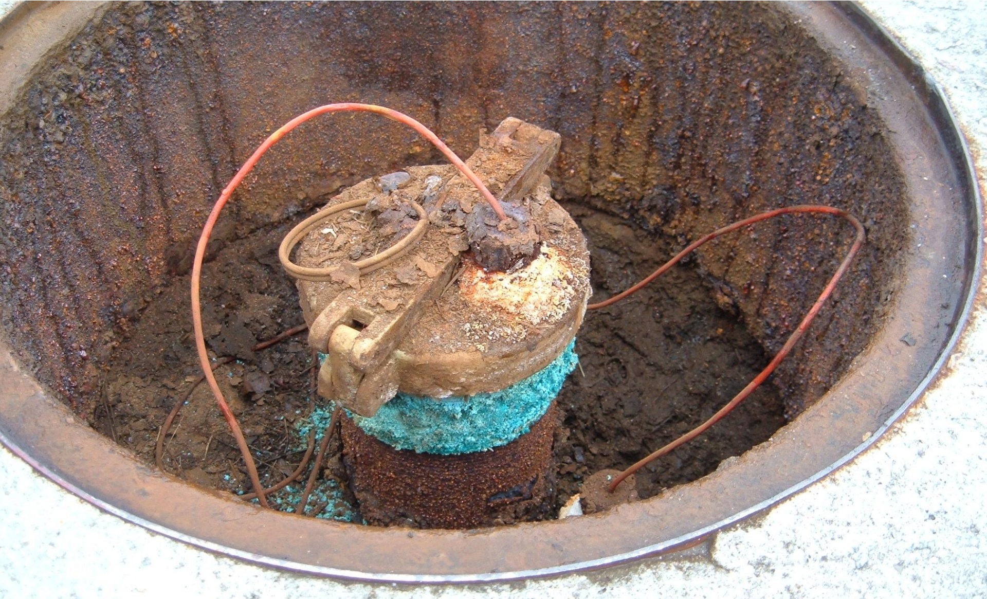
Evidence of vapor leaks
