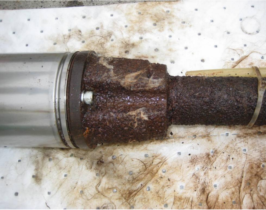
Submersible Pump & Riser (Left hand side is aluminum; Right hand side is steel)
