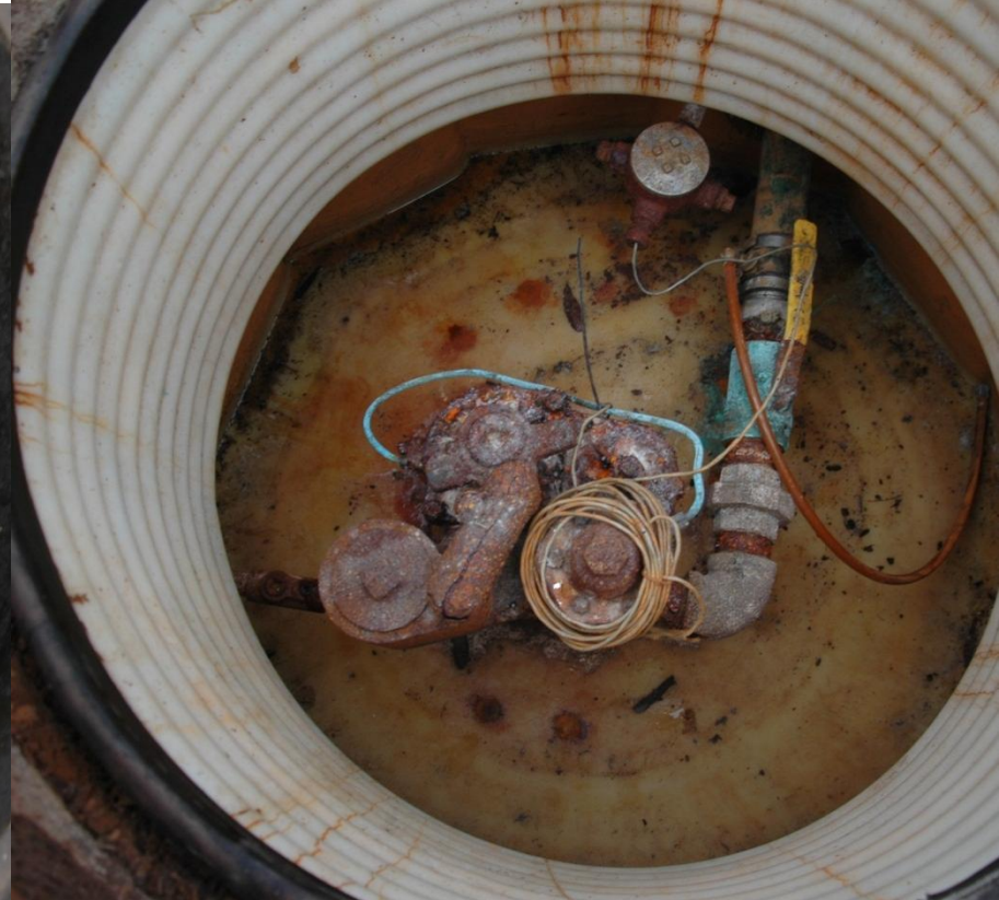
Regular Unleaded gasoline sump, same facility, Georgetown, South Carolina, November 2011
