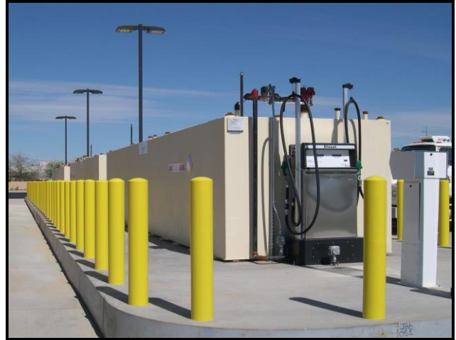
Hensley Distributing Refueling Facility
