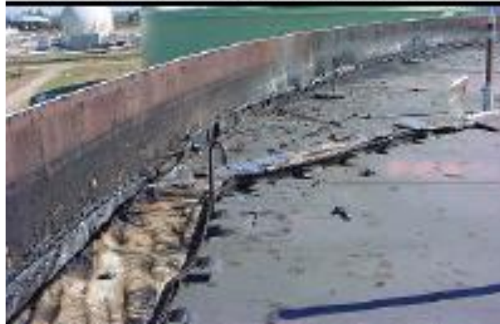
Seal Damage from Lightning-Related Fire
